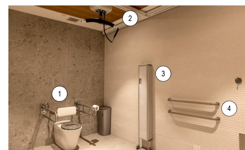
01_ ACCESSIBLE WC 02_ ROOM COVERAGE HOIST 03_ RETRACTABLE PRIVACY SCREEN 04_ CHANGING RAILS / CLOTHES HOOK
